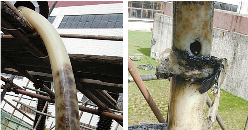
FIGURE 2. Left: Water tree caused by the interaction between the electric field and moisture. Right: Close-up of the mechanical damage to the insulation layer.
