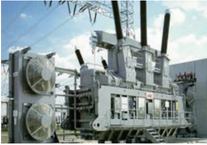
FIGURE 1. Photo of transformer equipment for high-voltage power lines.
